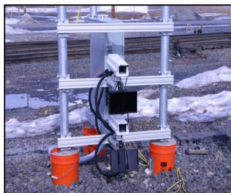
Figure 3: The BPMS module at the Selkirk installation
