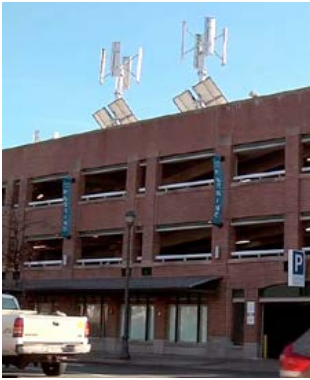
Verizon teamed up with Wing Power Energy to erect small wind/solar turbines on the roof of our building in Salem, Mass.
