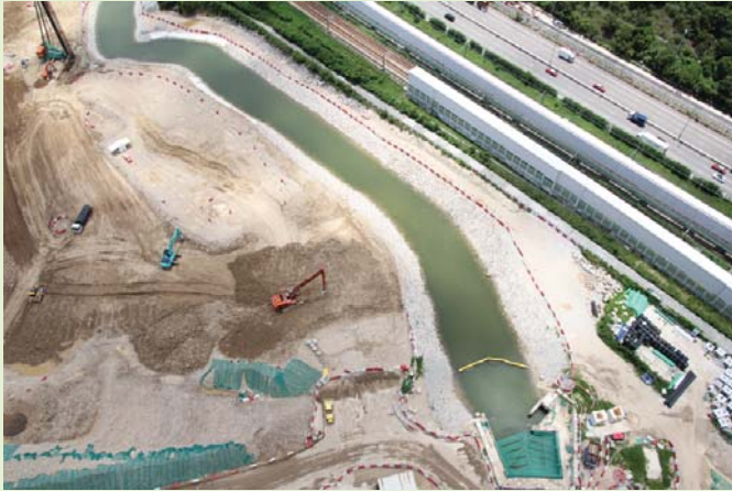
臨時排水渠道（已完成） Temporary drainage channel (completed)
