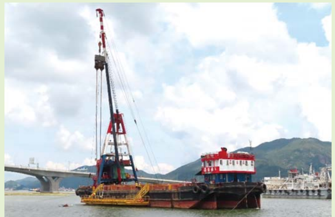
運用躉船安裝預制垂直排水板（進行中） Installation of prefabricated vertical drains by using a barge (in progress)
