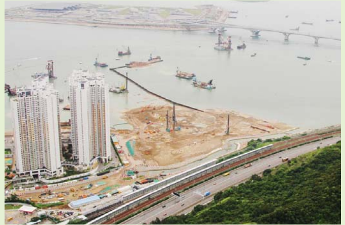
迎東邨對出的填海工程（進行中） Reclamation works outside Ying Tung Estate (in progress)
