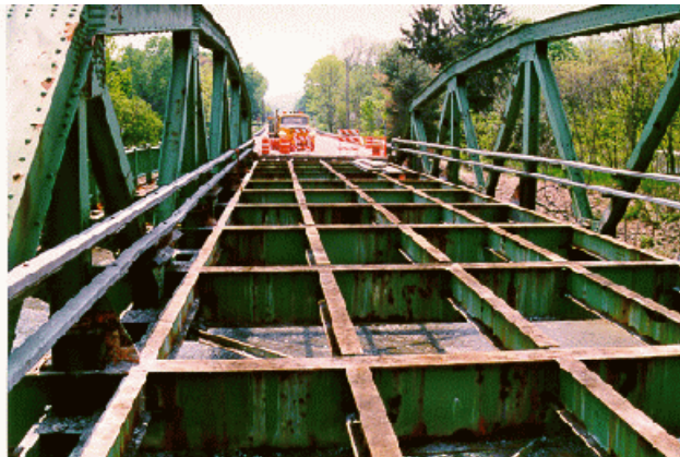
Figure 4. Corrosion of floor-beams.
