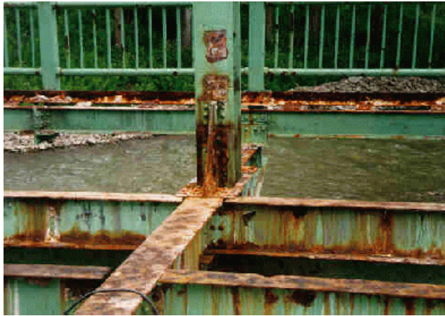
Figure 3. Corrosion at the floor-beam to truss connection.
