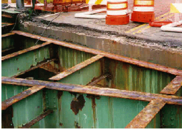
Figure 2. Corrosion of steel superstructure at the south abutment.
