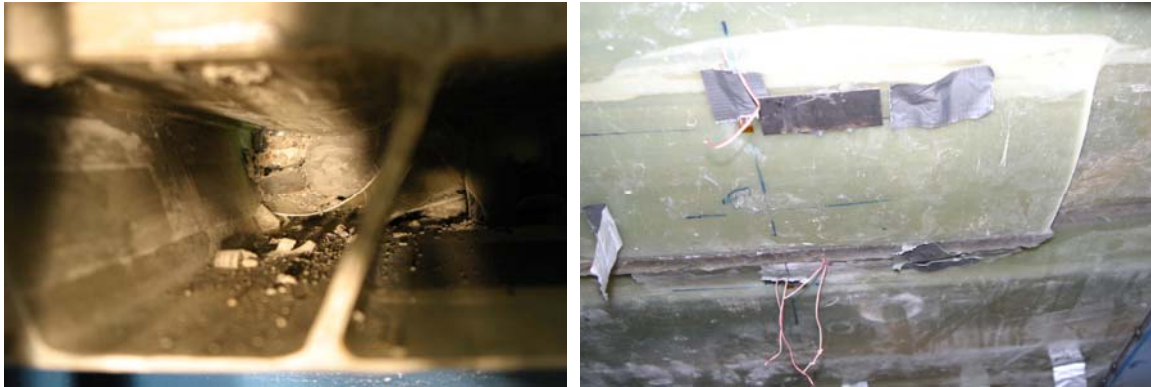
c. failure of inclined web
