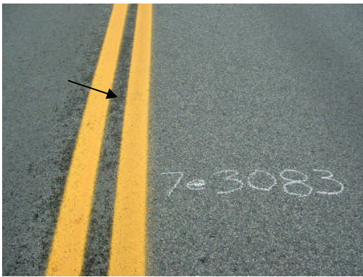
Photo 14: Ravelling Along Centerline – Route 7
