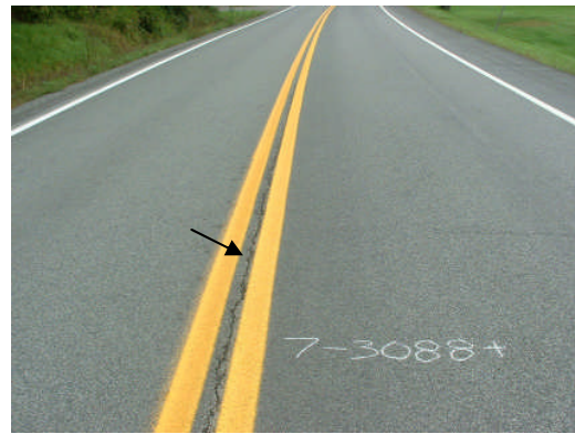
Photo 15: Cracking in Adhesive Section – Route 7
