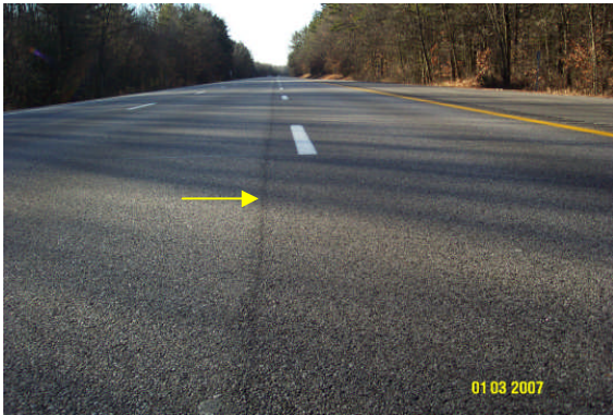
Photo 10: Crack in Control Section – I87
