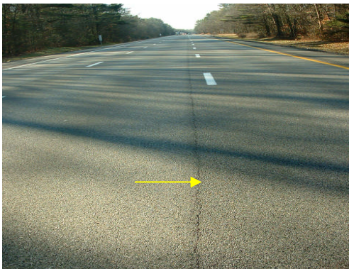
Photo 12: Crack in 4 inch Section – I87
