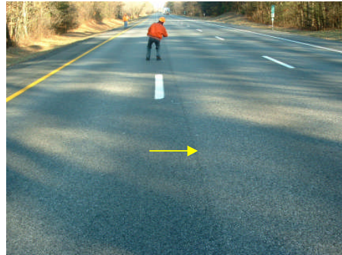
Photo 11: Crack in 2 inch Bead Section – I87
