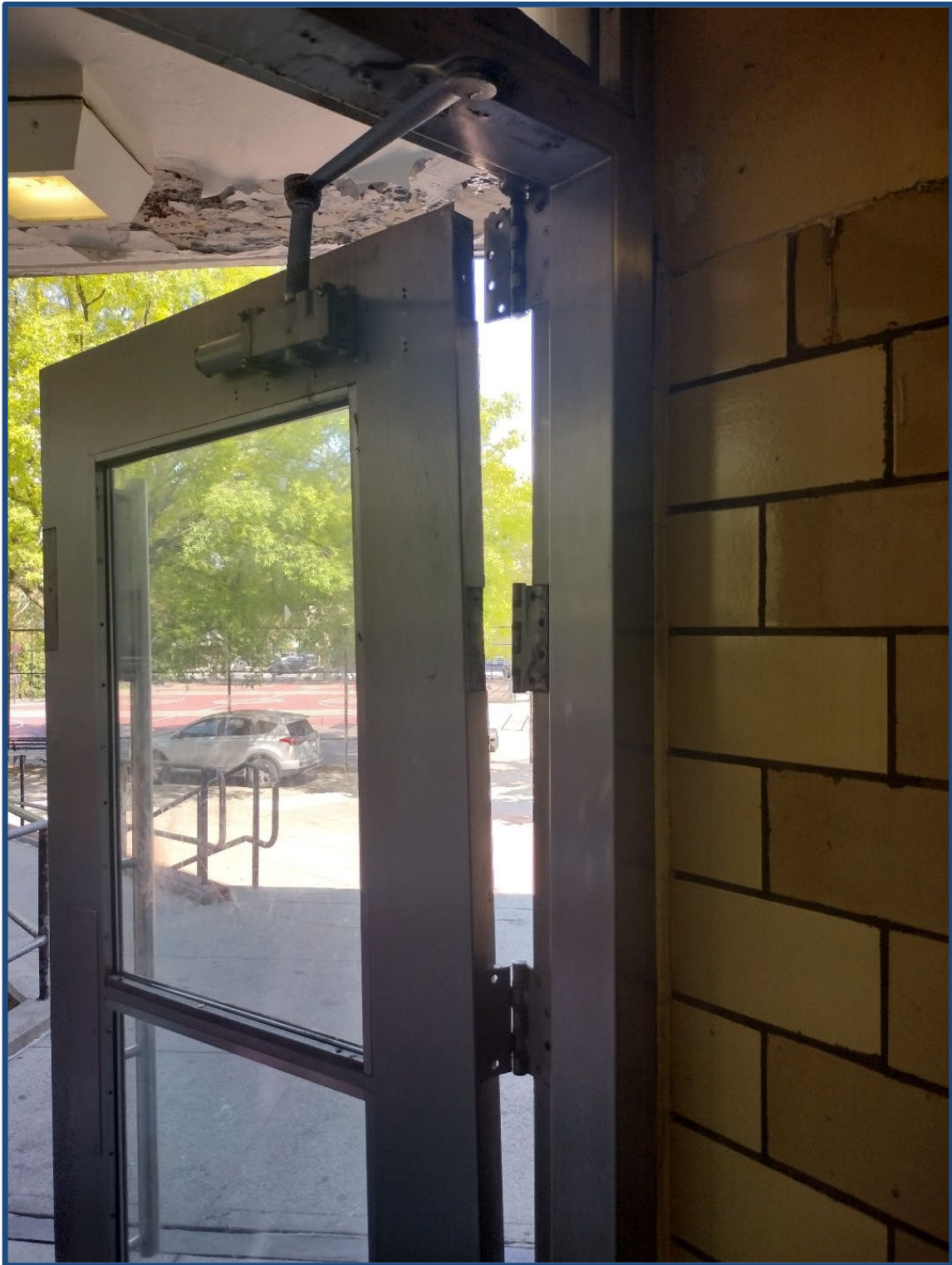
Damaged Door Hinge
