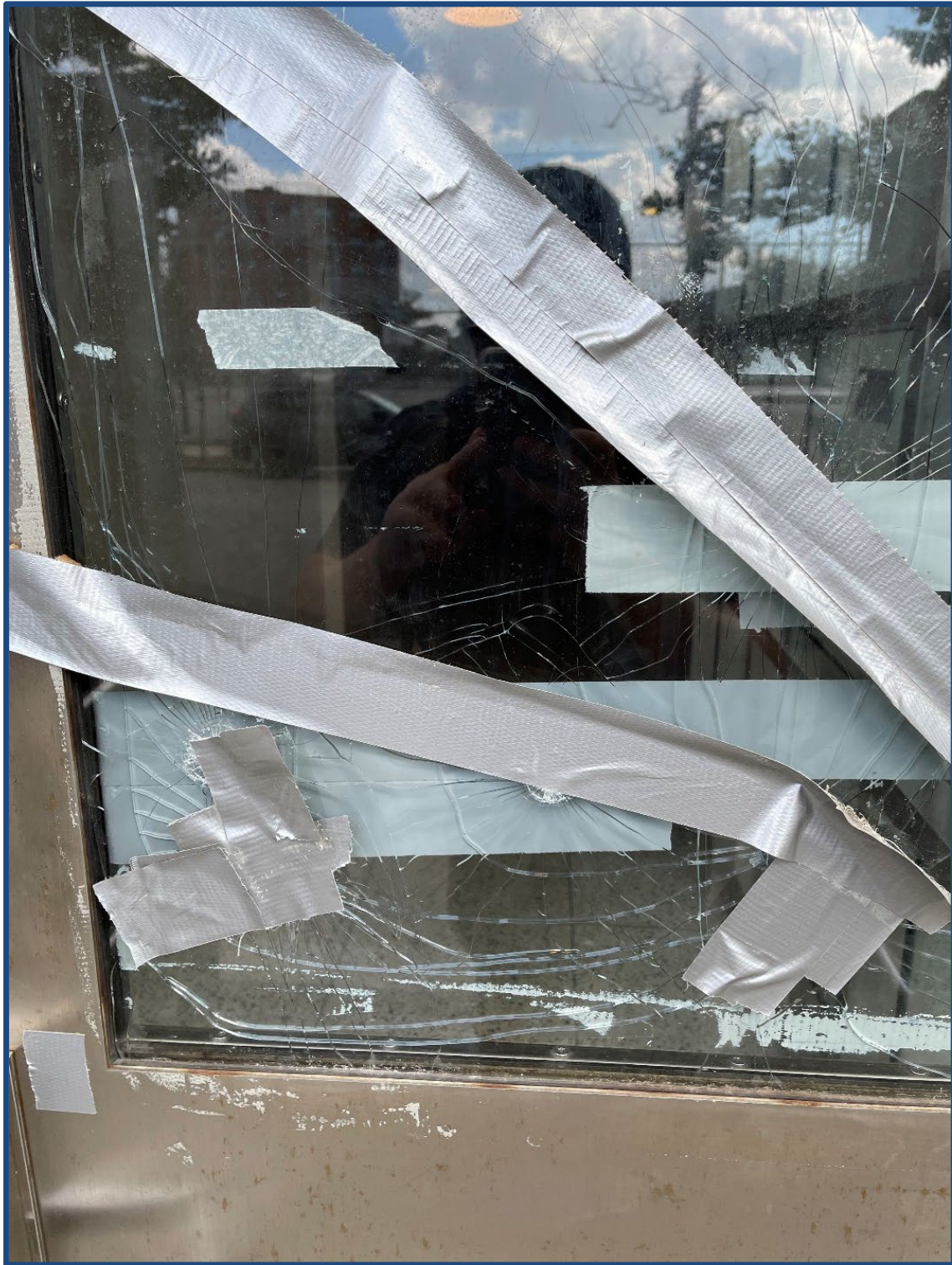
Damaged Door Window
