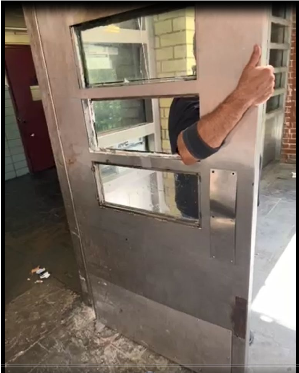
Missing Door Window
